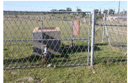
Riverlands BH No.3, fenced and locked
