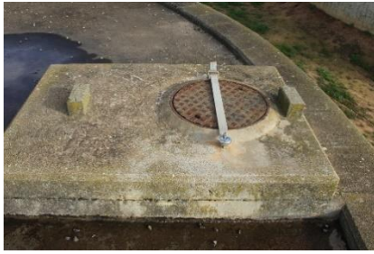
Wesbank Reservoir 0.988 MI, Cover locked.
