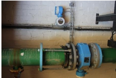
Moorreesburg Booster PS 200mm dia. Endress and Hauser bulk water meter
