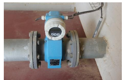
Tafelsig Booster PS bulk water meter
