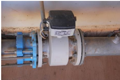
Abbotsdale Booster PS bulk water meter
