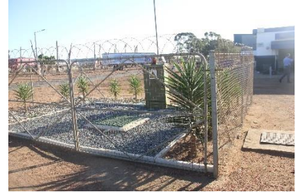
Darling Industrial sewer PS
