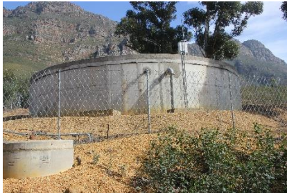
Riebeek Kasteel Reservoir No.2, 0.903 MI
