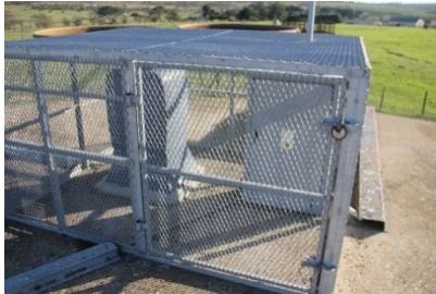
Chatsworth Reservoirs bulk water meters adequately protected in cage.
