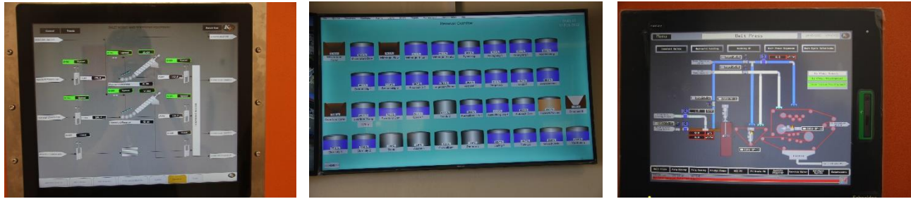
Moorreesburg WWTW: Scada for inlet works Reservoir levels of bulk distribution systems Darling WWTW: Scada system for Belt Press
